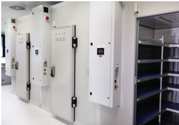
STABILITY ROOMS TURNKEY PROJECT BY ARALAB
