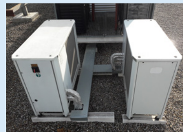
Back-up redundant systems
