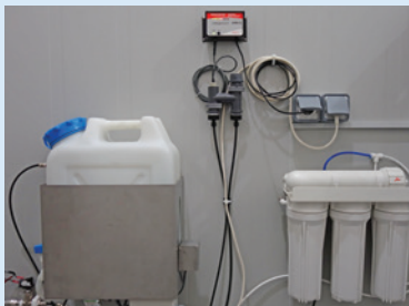
Water treatment systems
